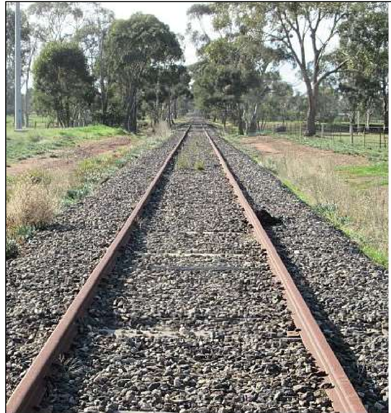
Atypical track condition as at March, 2022 on the Inglewood - Eaglehawk line. Line and top good, 47kg rail in long welded lengths fully base plated. Tie renewal required.
